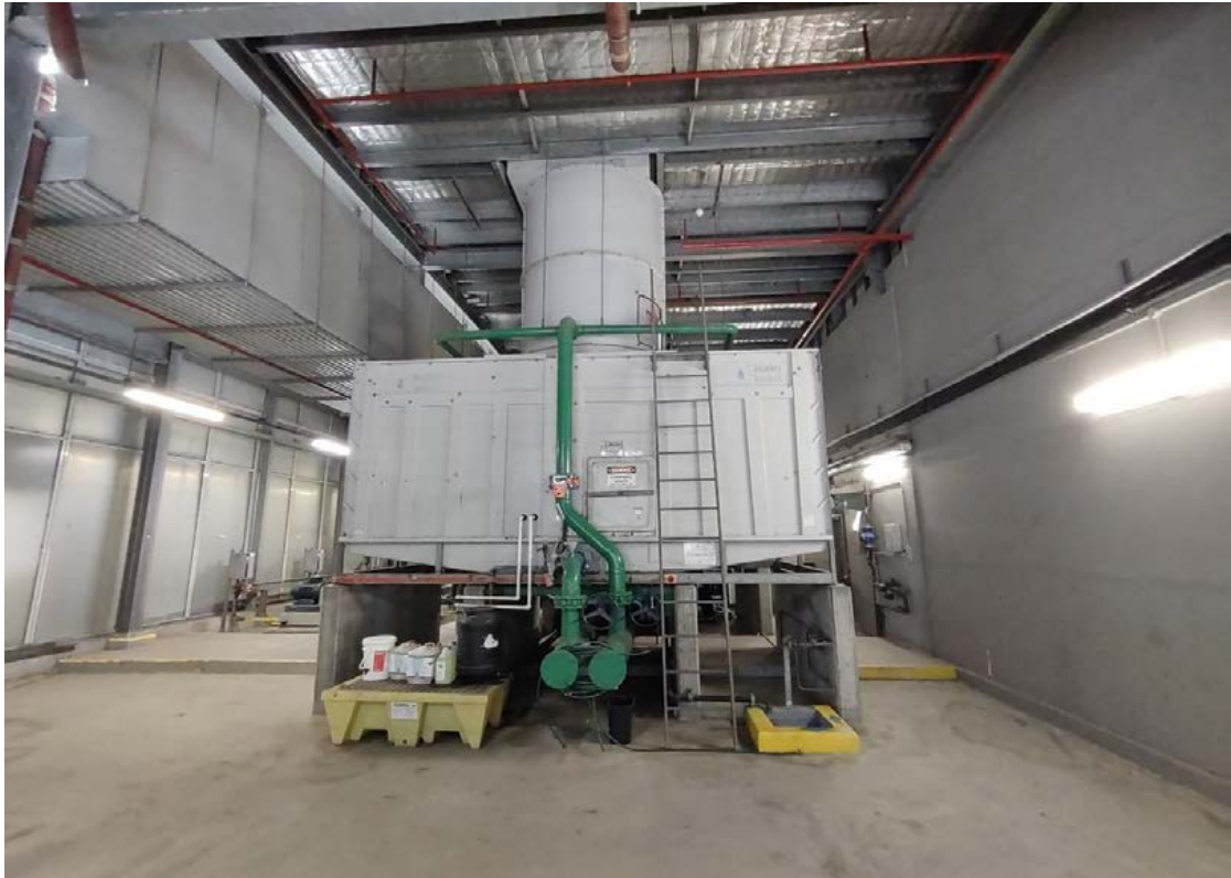
Photo 5: Coolin tower room in level 19
