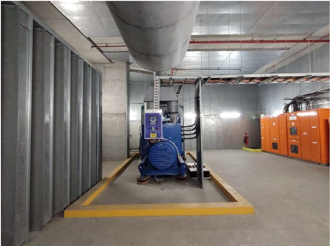
Photo 12: Diesel generator room in level 7
