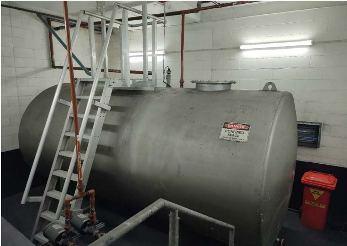
Photo 3: Above ground storage tank in basement 3 near Sussex Street
