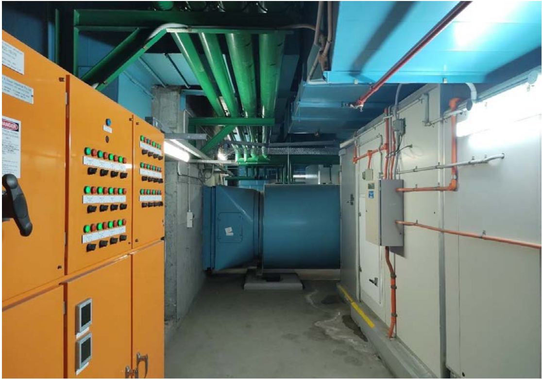
Photo 1: Plant room in level 19
