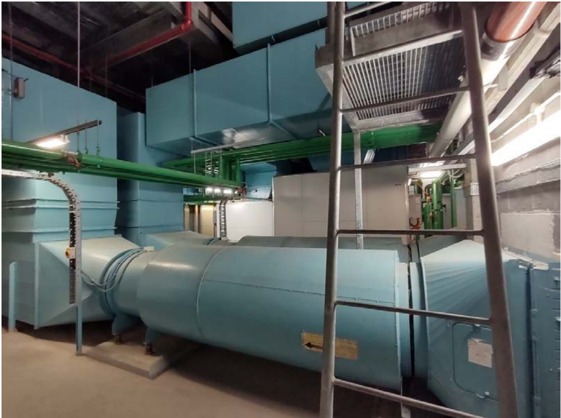
Photo 2: Plant room in level 7
