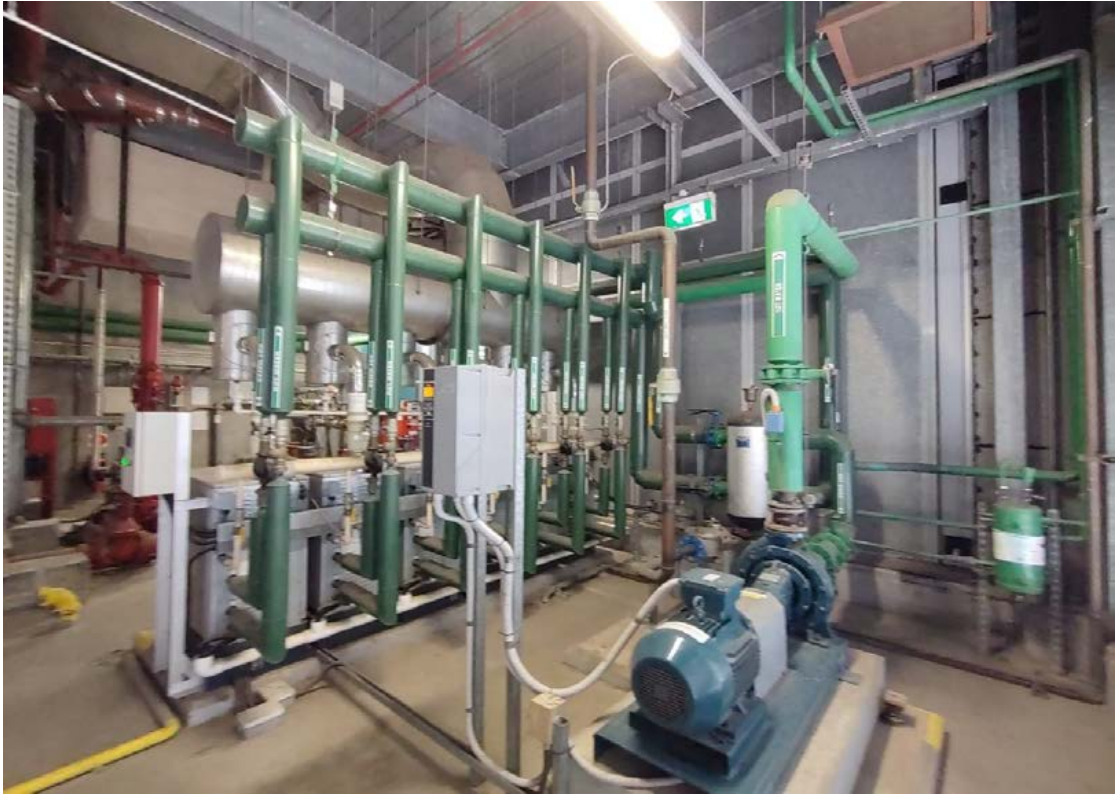
Photo 7: Lift motor room in level 20
