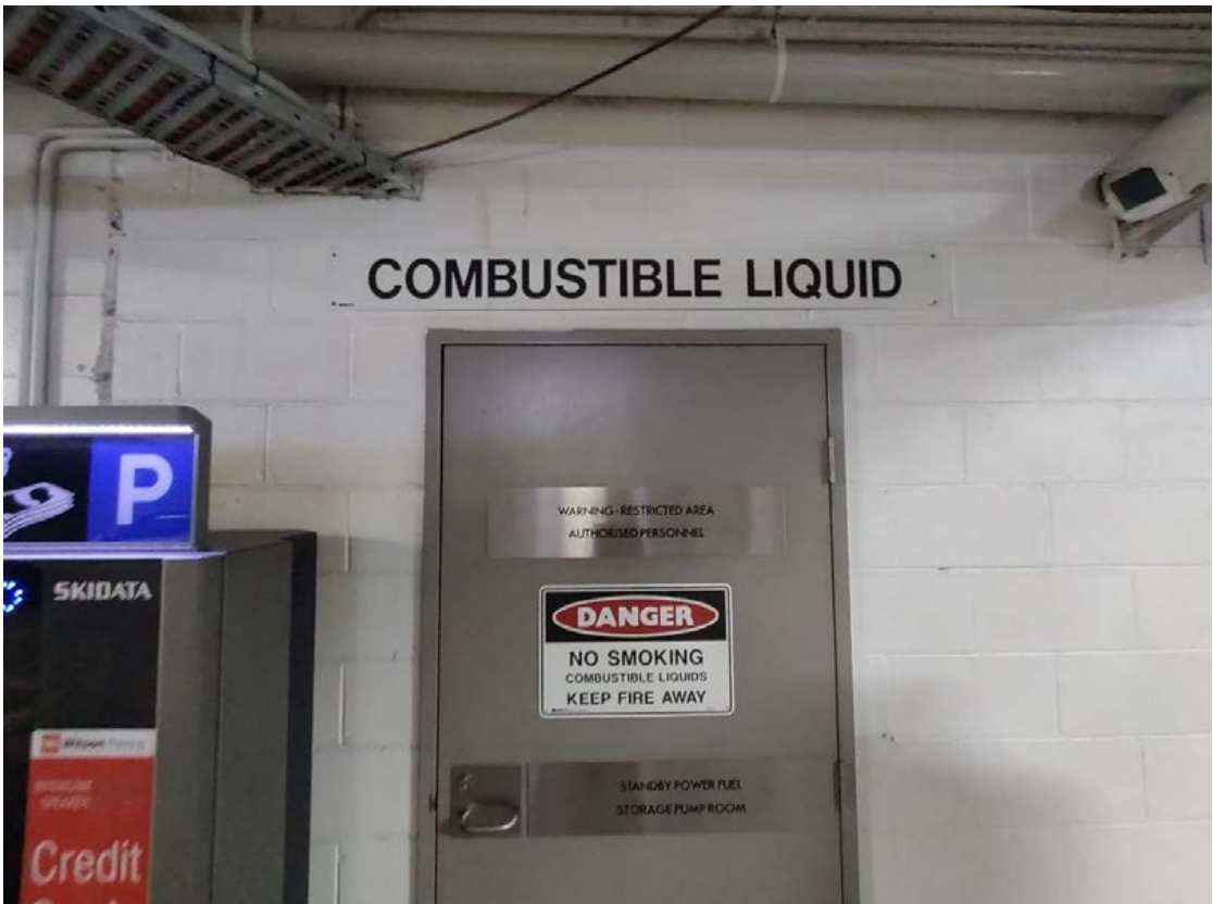
Photo 4: Standby power fuel storage pump room
